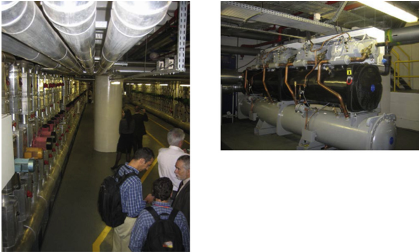
FIGURE 7.30 Cooling system driven by flat-plate solar collectors, commissioned in 2008, Lisbon, Portugal.
