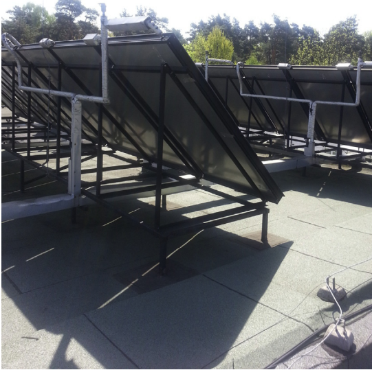
FIGURE 7.7 Solar collectors installed on supporting structures.
