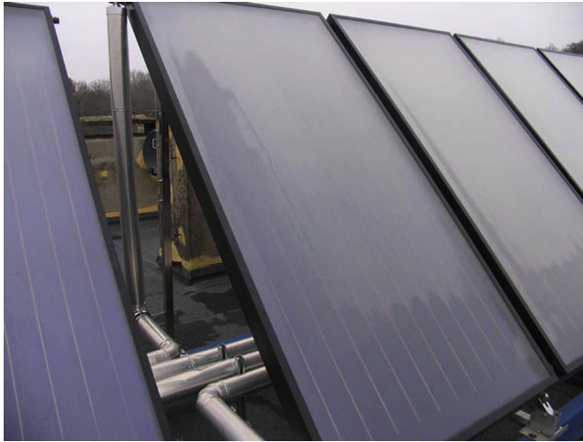
FIGURE 7.12 Solar collector with accumulated mist.
