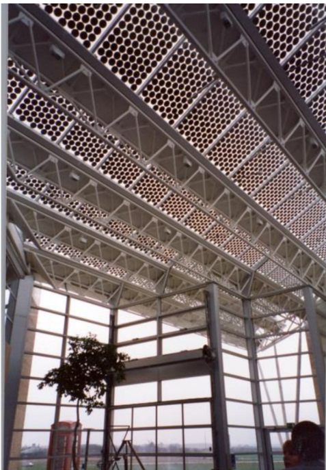
FIGURE 3.16 PV panel roof on a conference hall, Brundland, Denmark.
